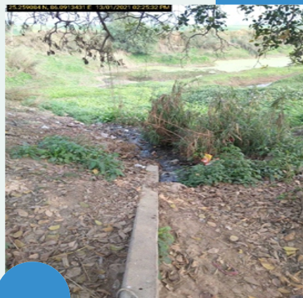
Wastewater Drainage BR_KUTHWA_243361_015011_W1
