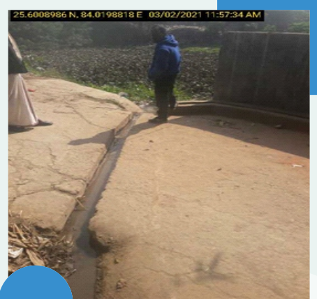
Wastewater Drainage BR_ARJUNPUR_247848_014324_W4
