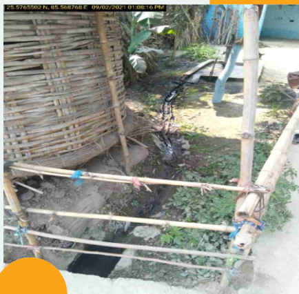
Wastewater drain BR_SARARI_231572_015421_W1
